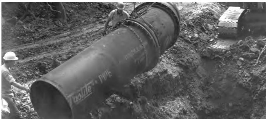
Installing a mechanical joint bend in a gravity sewer utilizing field-cut closure pieces to locate the fitting accurately.
